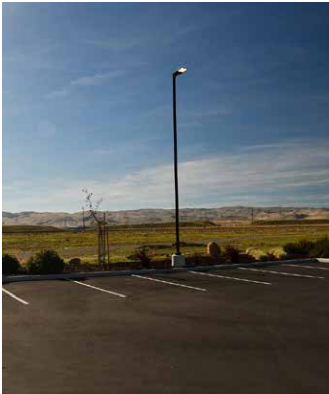
Typical parking lot lighting
