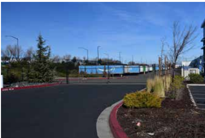
Gates visible from public areas are to be constructed of tubular steel or similar material
